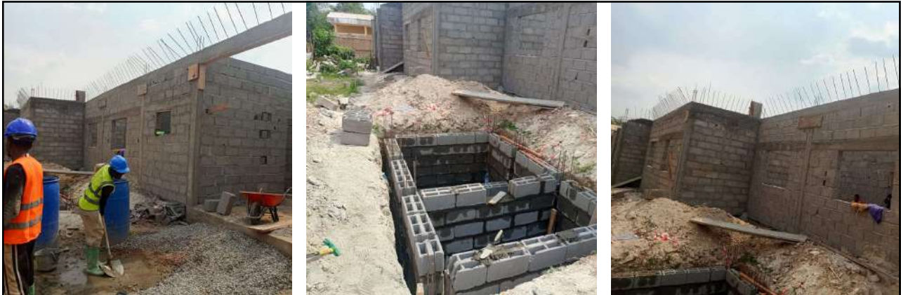
• Construction of an imaging center at the Mamfe District Hospital Supply and installation of digital Radiography System with Accessories; Supply and installation of furniture ; construction of Solar Farm, Manyu, Southwest
